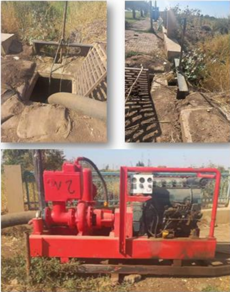
Fig.5 Outlet discharge and the pump used.
